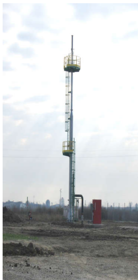
Example of Vent stack with snuffing system
